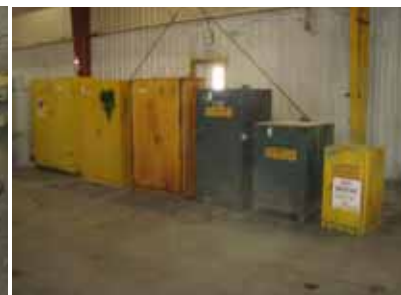
Flammable Liquid Storage
