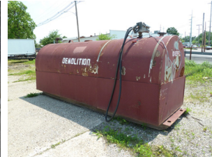
Fuel Storage Tank
